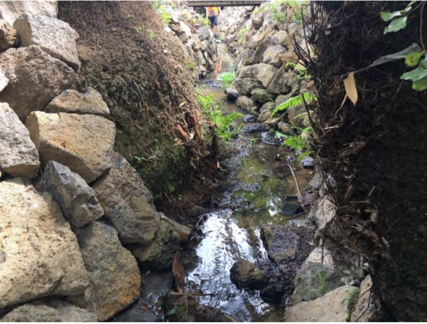
A reach of Mission Bay Stream through residential properties with riprap as bank lining (MIS_TRIB4_3).
