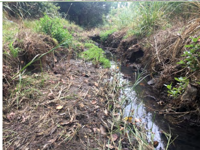
Mass wasting and slumping in the channel (Tributary ID: KOH_MAIN_10). Floodplain could be enhanced for inanga spawning habitat.
