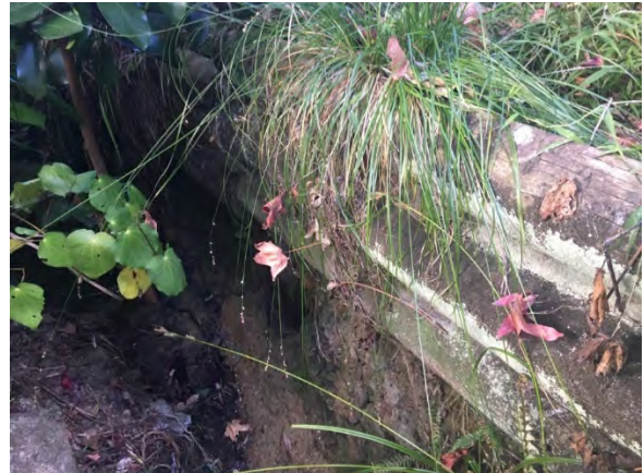
Bank lining at 18a Godden Crescent on private property (MIS_TRIB5a_1) (UNK_009).
