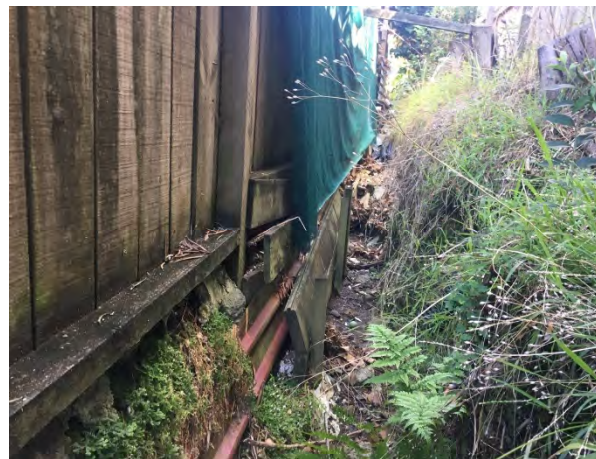
Haphazard bank lining encroaching on a nearby shed (STH_TRIB4_4) (UNK_056).
