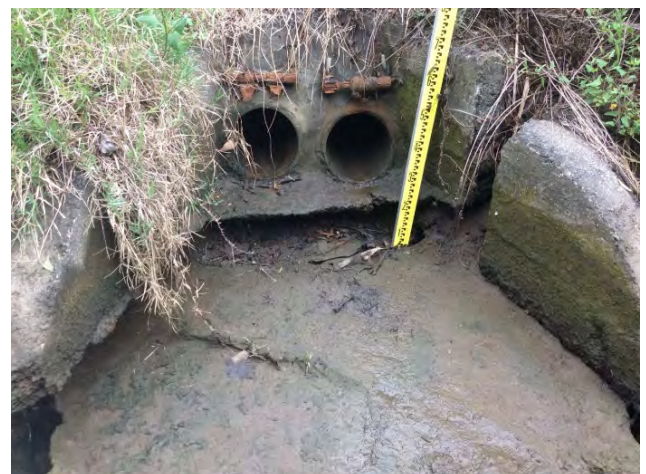
Outlet with detached wingwall, apron and snapped off tide gates (2000799090).
