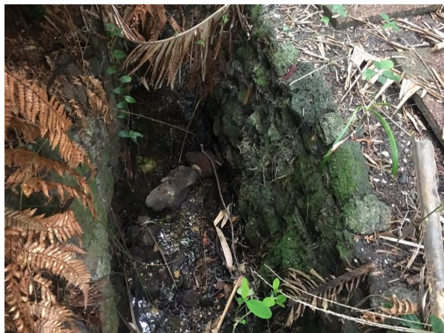
Approximately 70 m of Karaka Bay Stream is lined with concrete and rip rap (KAR_MAIN_1).
