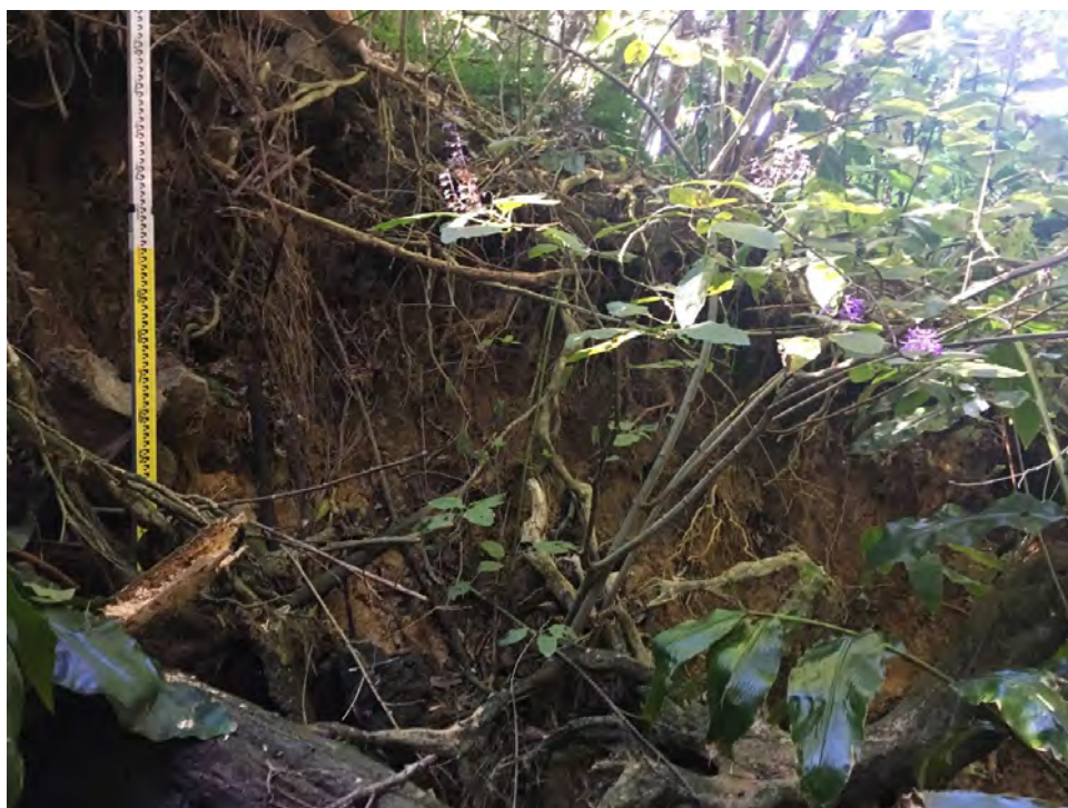
Figure 32. The erosion hotspot at KOH_TRIB7a_1 is associated with the stormwater outlet (Asset ID: 2000130324) shown on the top left-hand corner of the image.
