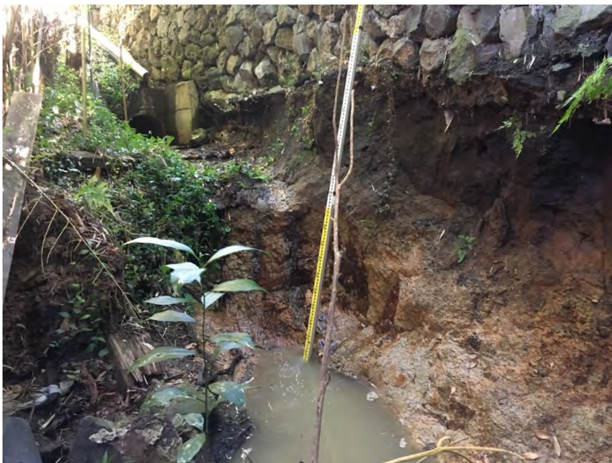
Figure 33: Erosion associated with under the retaining wall at 27 Geraldine Place along KOH_TRIB3a_5.
