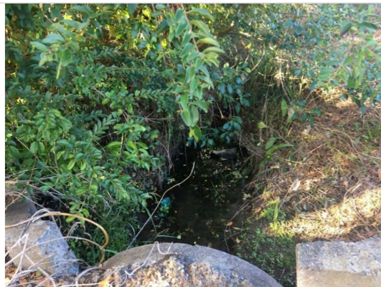
Outlet at the top of stream (SAP ID: 2000077826, 2000077826) showing low banks and poor vegetation.
