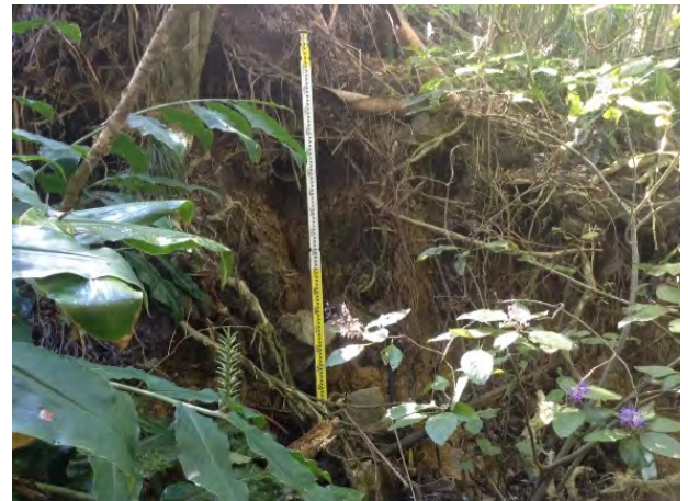
The dissipation structure for the outlet at 92 Allum street (2000565387) has completely fallen away due to erosion.
