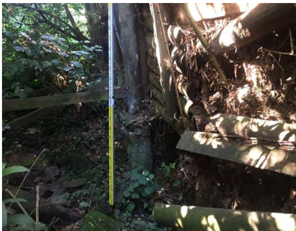
Bank lining undercut at 2/21 Geraldine Place (KOH_TRIB3a_5) (UNK_038).
