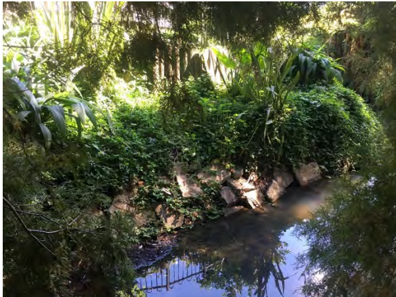
Bank lining in Churchill Park (AC land) (UNK_004) made up of poorly placed concrete blocks and gabion baskets.
