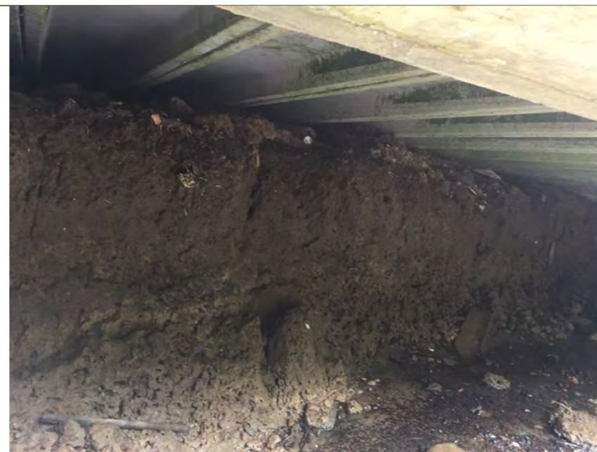
Undermining occurring the wall under the parking garage structure at 29 Tamaki Drive.
