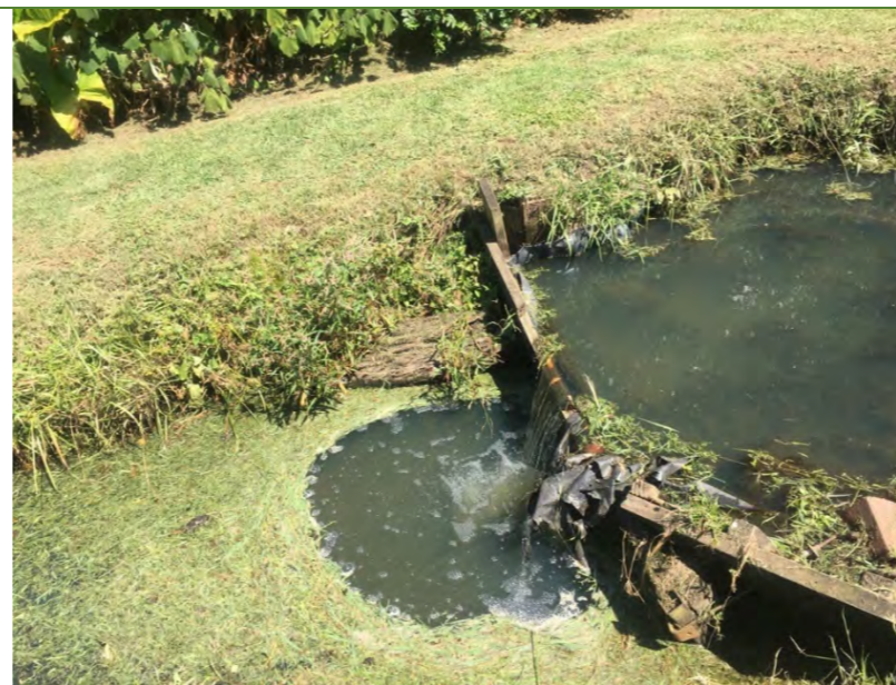
Multiple ad-hoc weirs and dams structures used to create ponding sections of stream.
