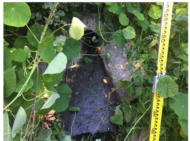
Informal concrete outlet at 23 Tarawera Terrace is undercut and may fall into stream channel (2000780248).
