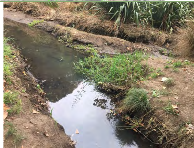
Erosion where the flows from the outlet (asset ID: 2000229311) hit the adjacent bank.
