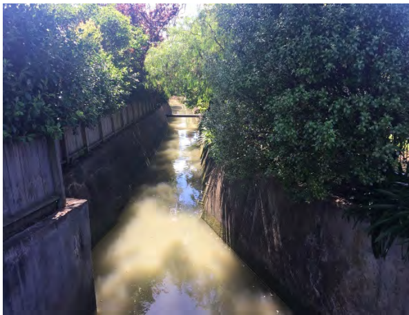
The coastal reaches located along KOH_MAIN 1 to KOH_MAIN_4, Mission Bay sub-catchment stream mouth are concrete lined with narrow riparian margins.
