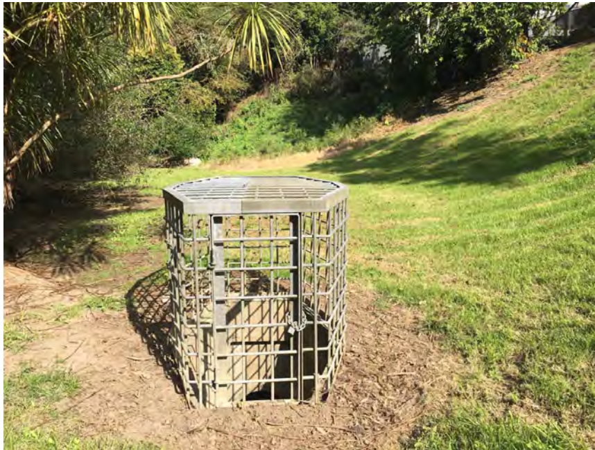
Figure 23: Dry Detention Pond located near (Tributary ID: KOH_TRIB6_1) constructed for stormwater management. The Council stormwater asset is located adjacent to private residential properties.
