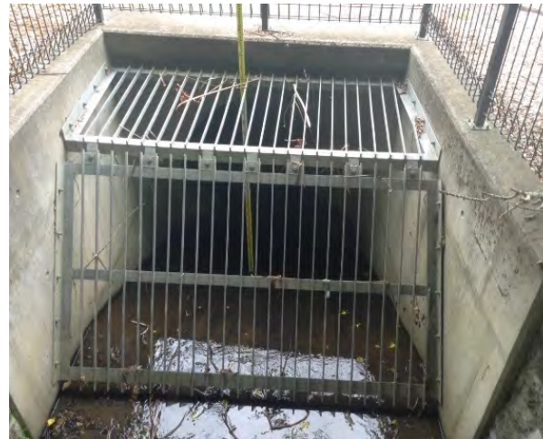
Auckland Council owned inlet in Dingle Dell reserve (DIN_MAIN_2, 2000919661). A steep concrete ramp into the inlet was causing a barrier to swimmers.
